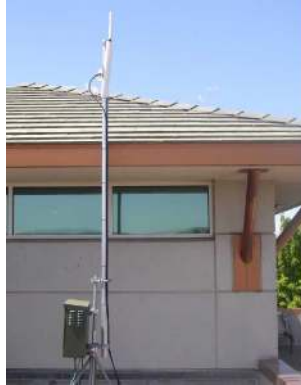
Figure 4. Example Installation on Building Rooftops
