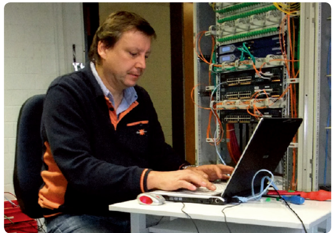
Frank Weirauch, Lead Telecommunications Engineer with the Saxony Highway Authority
