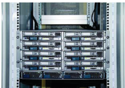
Cisco Unified Computing System
