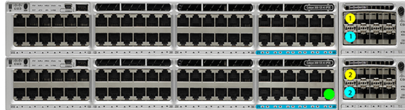
Dual 10/25GE ToR Switches (standalone or stacked)
