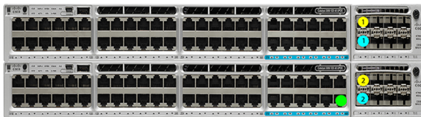
Dual 10/25GE ToR Switches (standalone or stacked)
