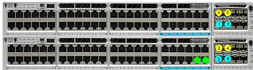
Dual 10/25GE ToR Switches (standalone or stacked)
