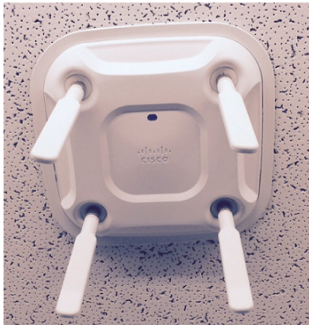
Figure 9-2 AP With Antennas Arranged (correctly) in Same Orientation
