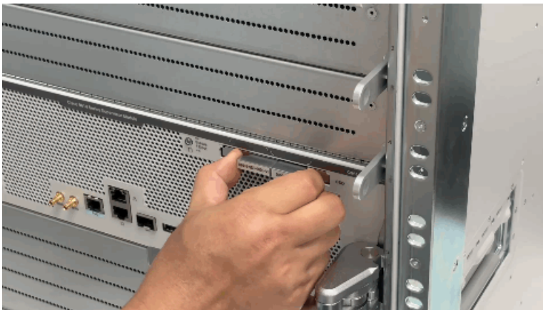
Figure 14: Removing the SSD from the supervisor
