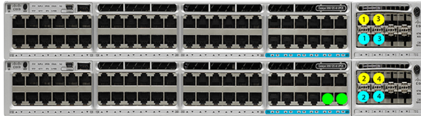
Dual 10/25GE ToR Switches (standalone or stacked)
