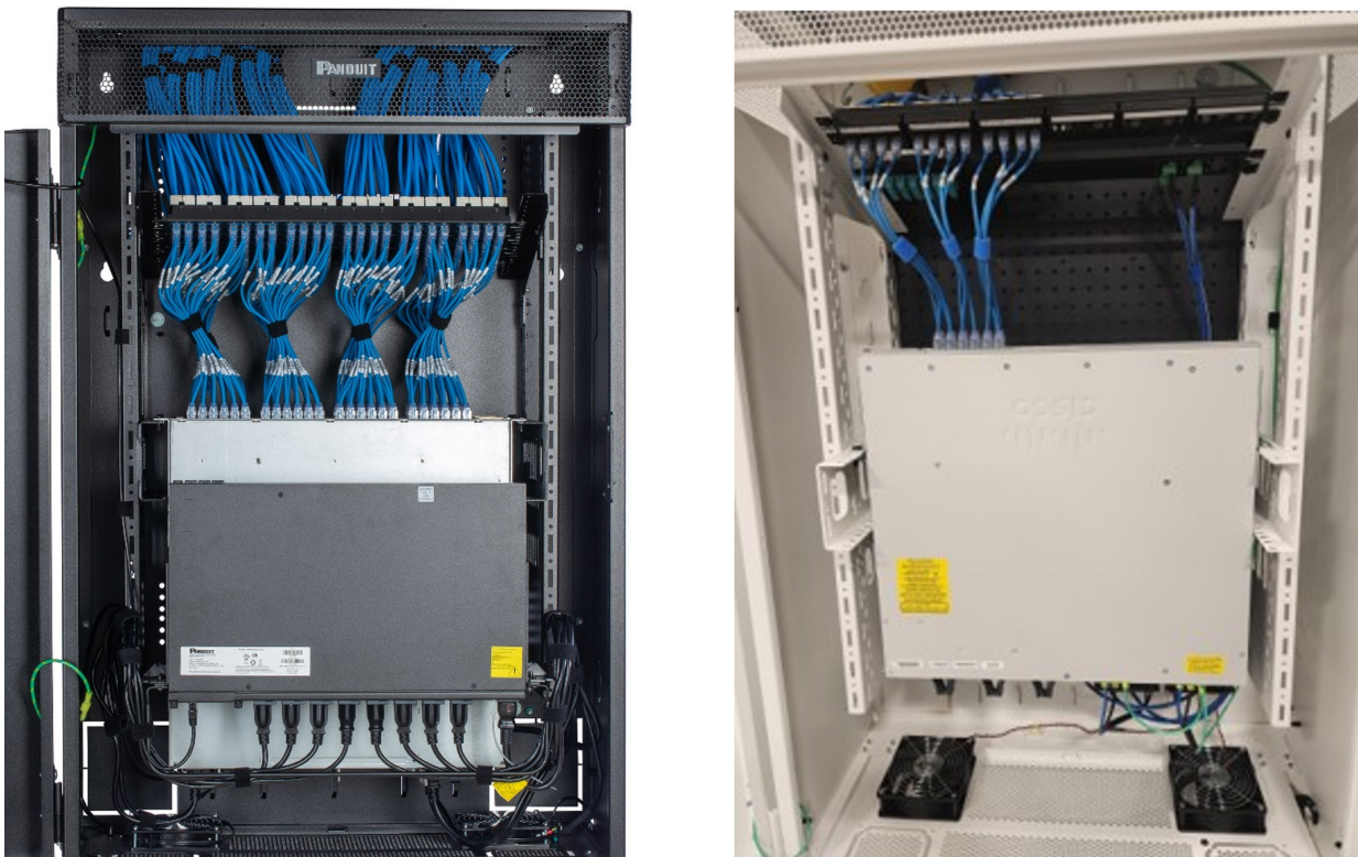
Figure 38. Cisco Catalyst 9300 deployed in Panduit TrueEdge
