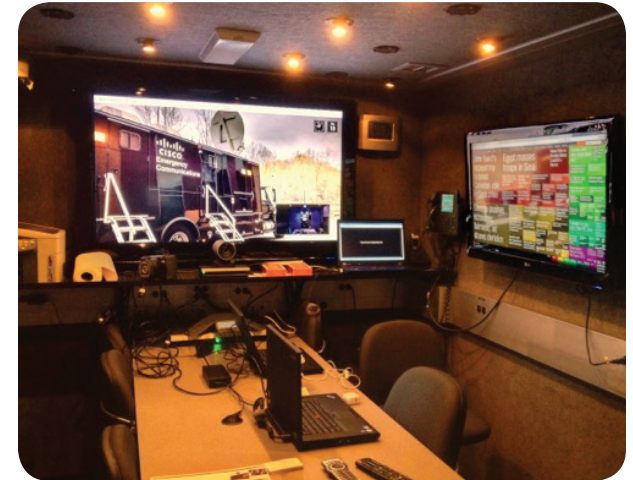
Figure 3: The Cisco NERV conference room enables decision makers to manage crises with a range of voice, video, radio and data communications at their disposal.
