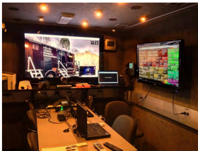
Figure 3: The Cisco NERV conference room enables decision makers to manage crises with a range of voice, video, radio and data communications at their disposal.
