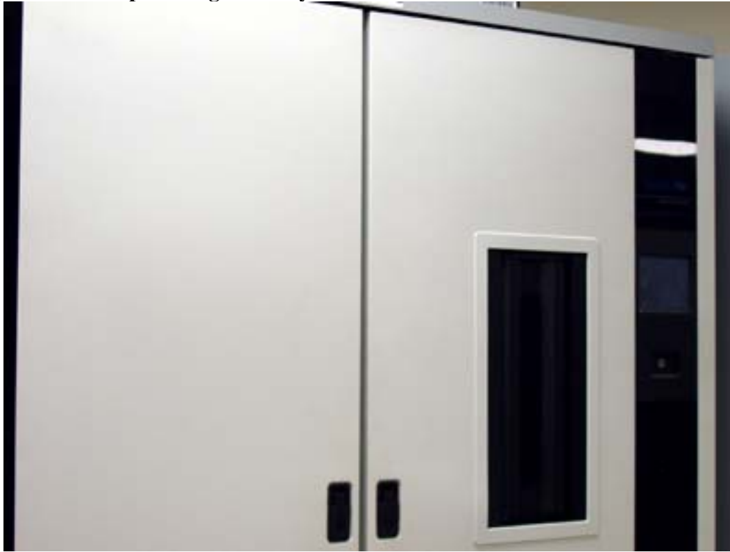
Figure 3. Tape Storage Library
