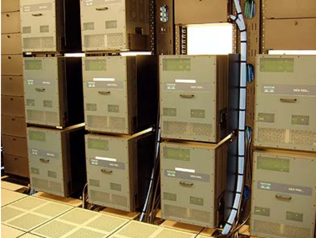
Figure 1. Storage Switches in the Data Center
