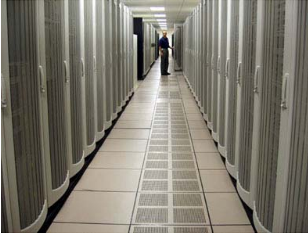
Figure 4. Rows of Servers in the Data Center
