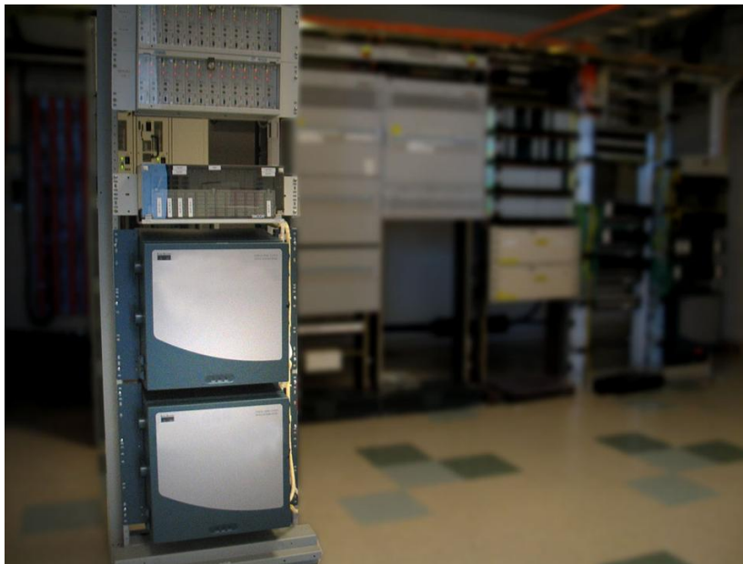
Figure 4. Legacy Infrastructure (Background); Cisco ONS 15454 Infrastructure (Foreground)
