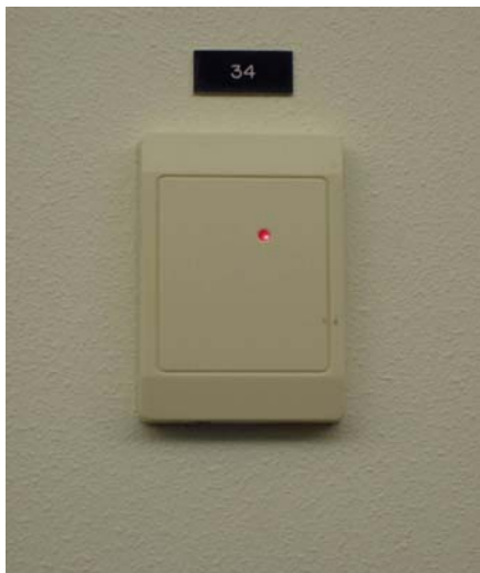
Figure 4. Proximity Badge Reader
