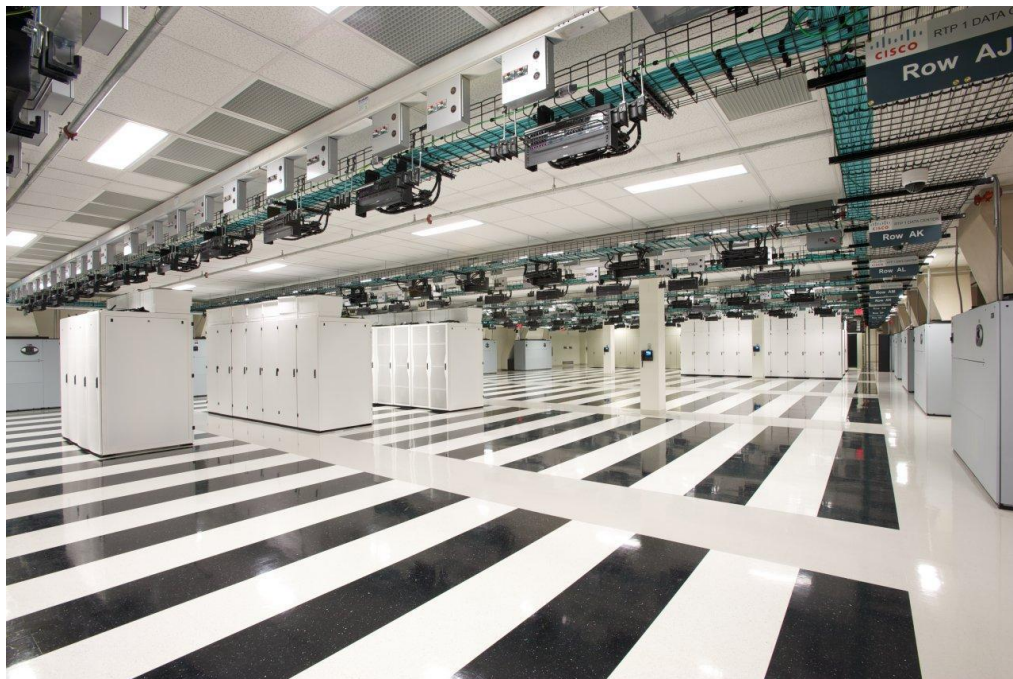
Figure 4. Cisco Data Center – Raleigh 1 Does Not Have Raised Floors, and Overhead Cabling Simplifies Changes
