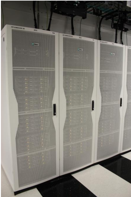
Figure 2. High-Density Computing Conserves Floor Space in Cisco Data Center – Raleigh 1
