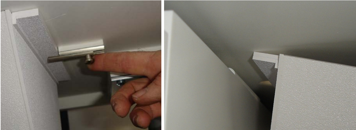
Figure 1-26 Open Cable Trough
