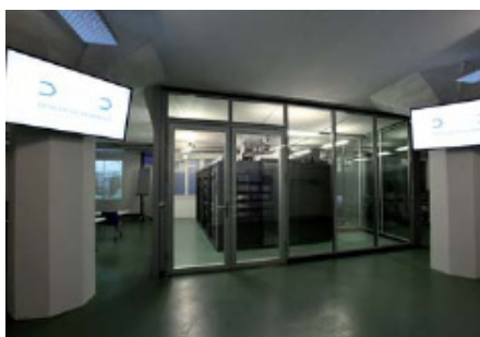
At the Datacenter On Demand in Zurich, about 70 percent of server space was saved.
