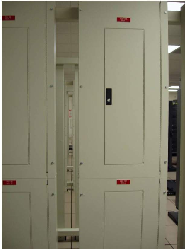
Figure 35. Power Distribution Cabinets
