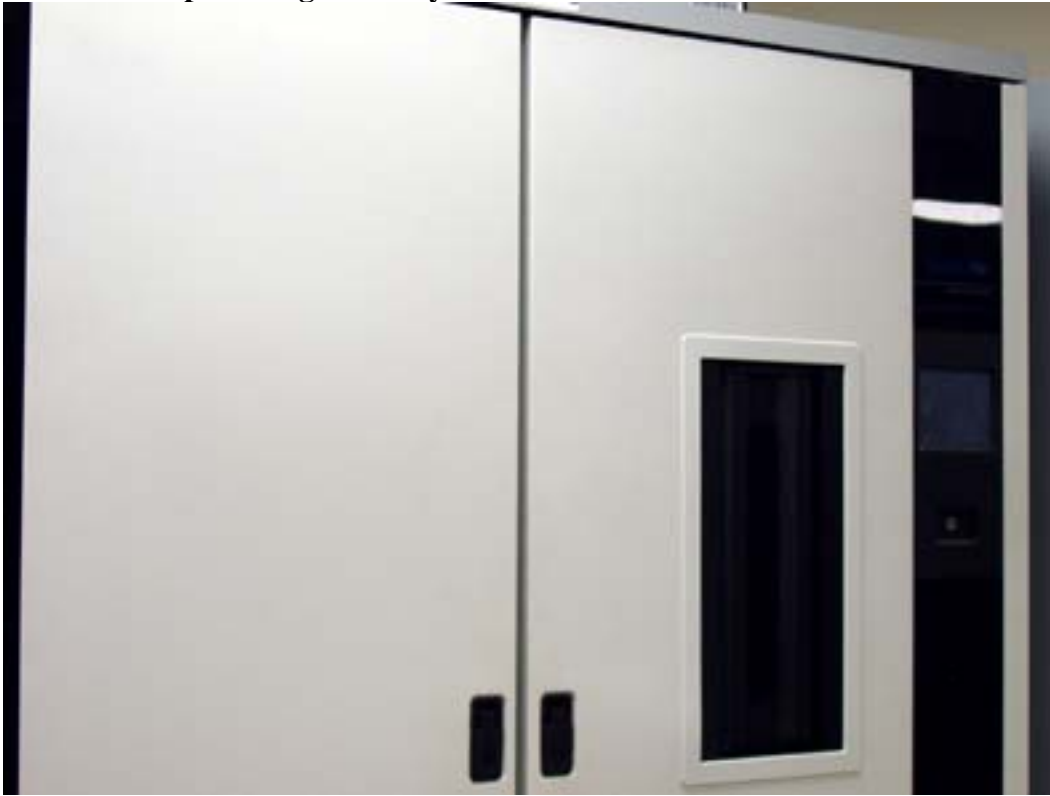
Figure 29. Tape Storage Library
