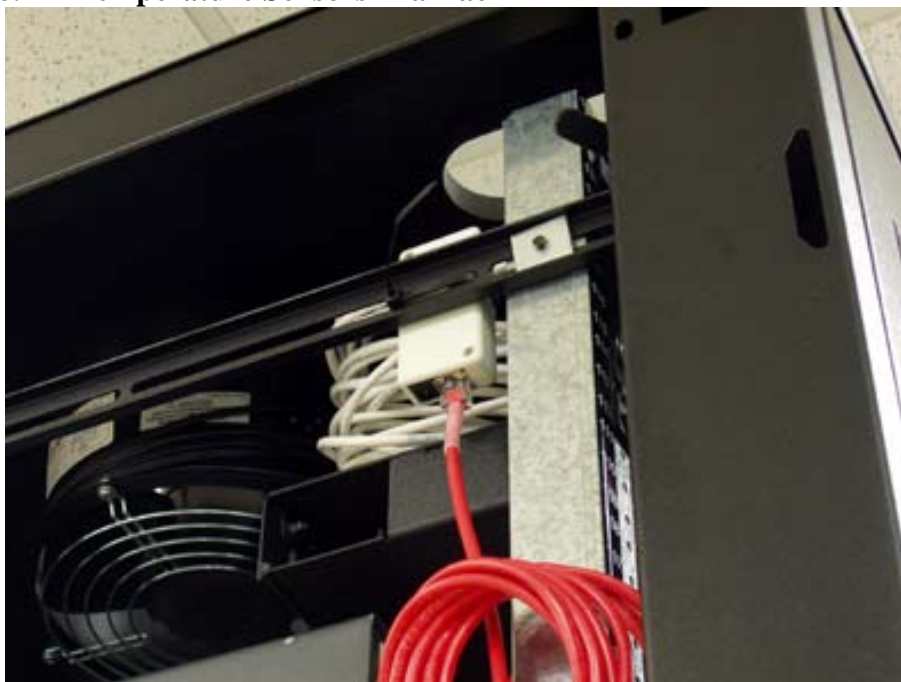
Figure 38. Temperature Sensors in a Rack
