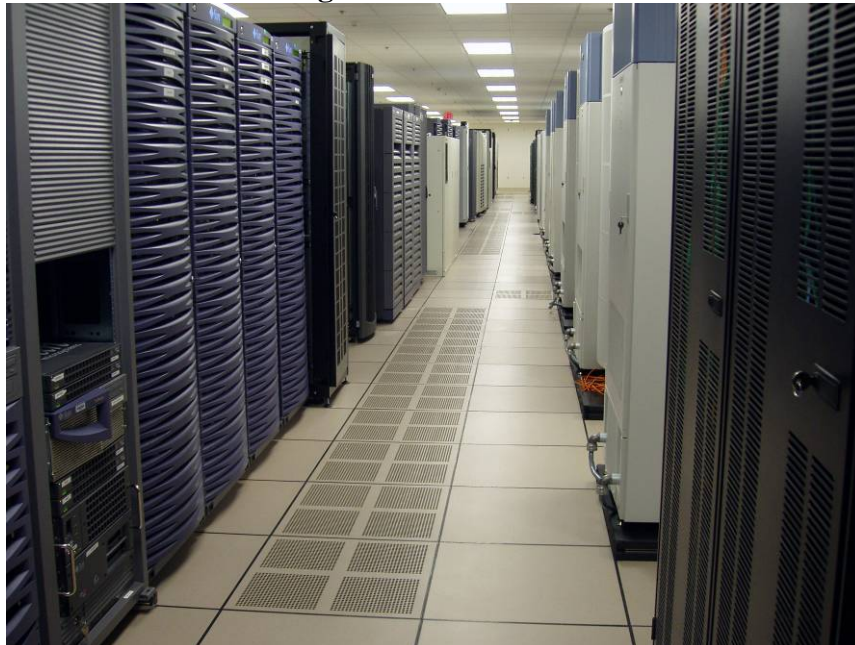
Figure 39. Server Racks Facing Each Other
