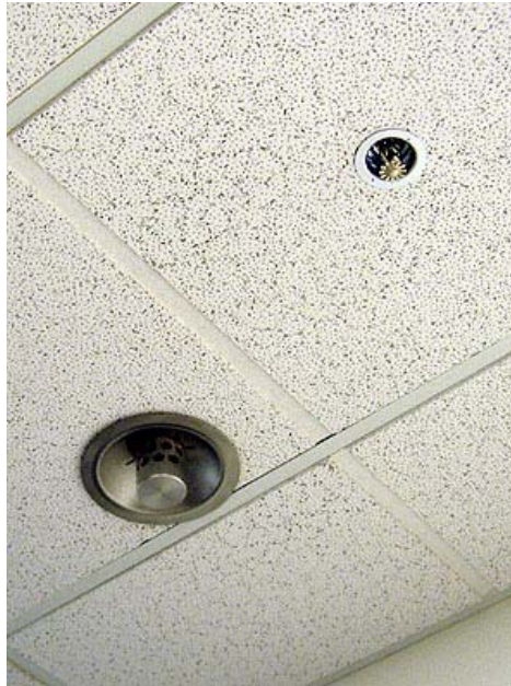
Figure 41. FM200 and Water Nozzles in the Ceiling
