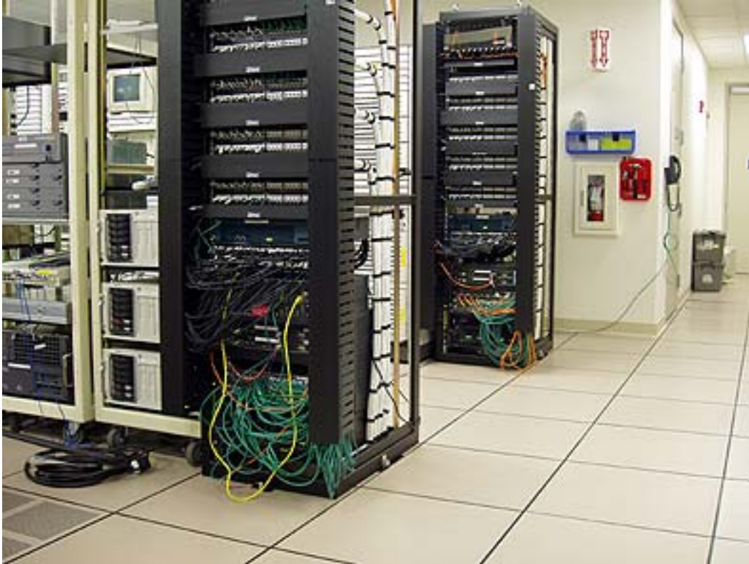
Figure 26. Network Rack at End of Half-Rows
