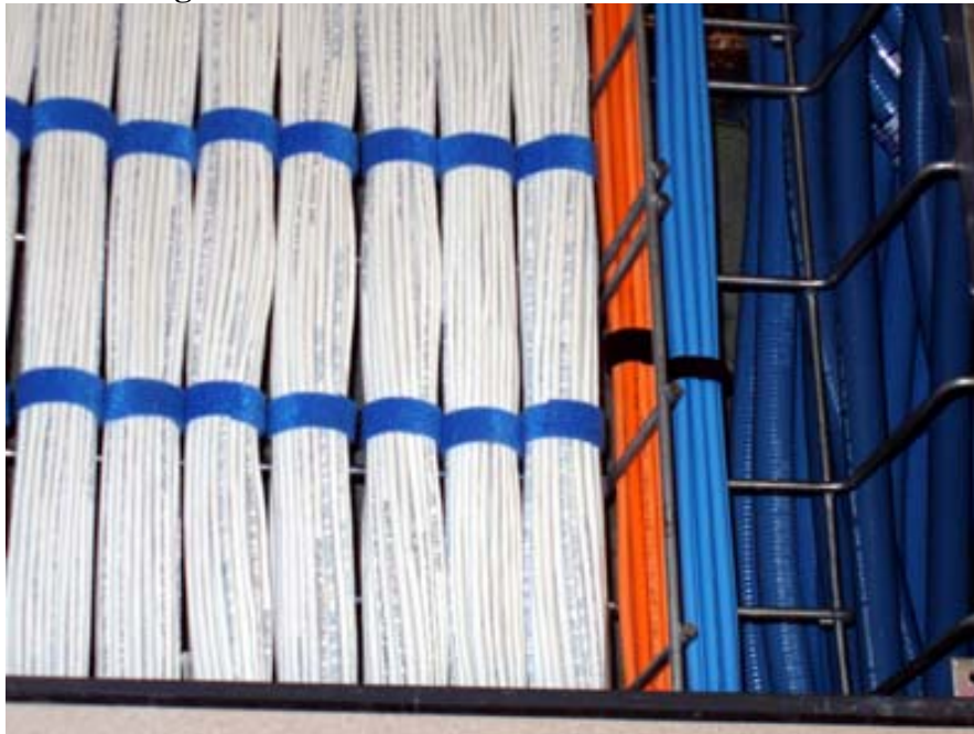
Figure 36. Cabling Under the Floor
