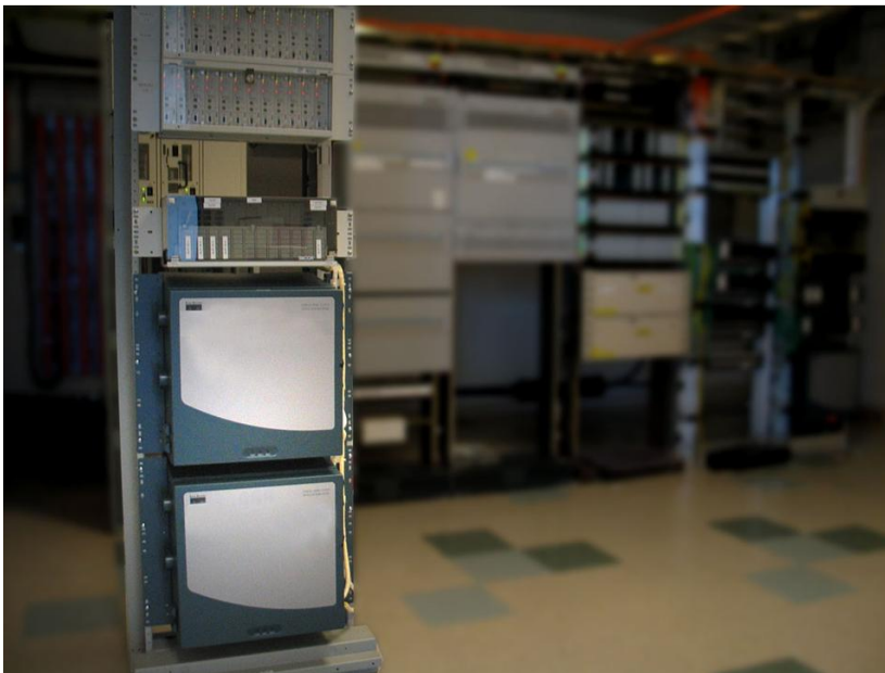
Figure 4. Legacy Infrastructure (Background); Cisco ONS 15454 Infrastructure (Foreground)
