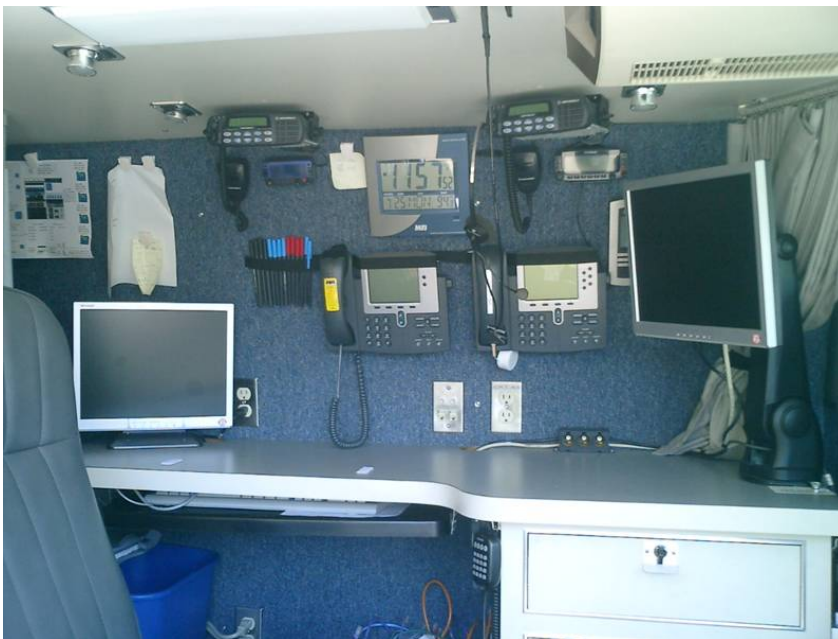
Figure 2. Dispatchers at the Security Operations Center Can Manage Talk Groups, Including Participants with Radios, Wireline Phones, Cellular Phones, and PC Clients
