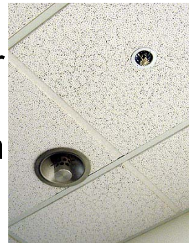
Water and FM200 Nozzles
