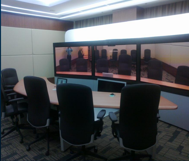
TelePresence Room at MAMPU Cyberjaya
