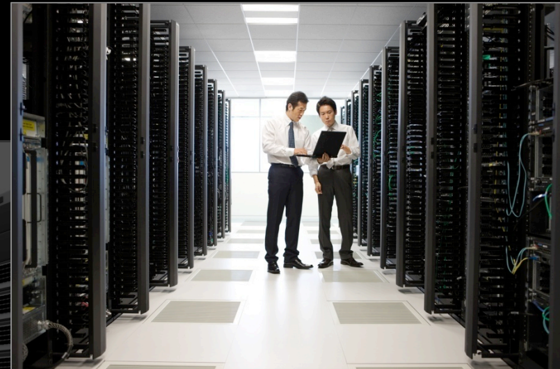
Provider of Server Room
