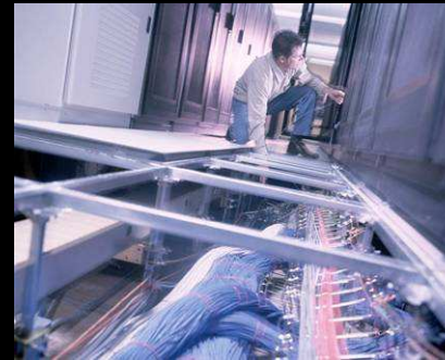
Core and Distribution
