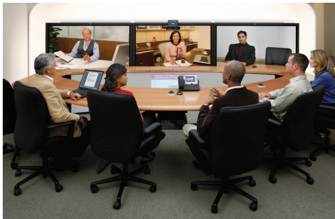
Cisco TelePresence 3000 13 units
