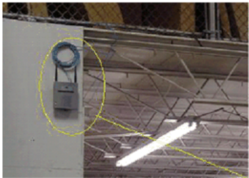
Figure 12 AP and Antennas Mounted on a Wall, away from I-Beams
