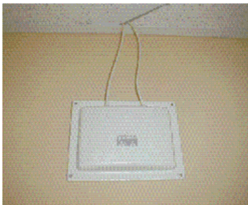
Figure 17 Aironet 2012 Antenna Mounted to a Wall
