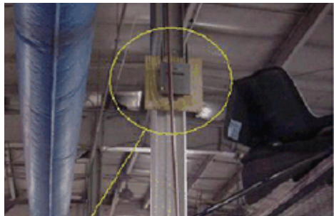
Figure 10 Improper Placement of Antennas Near an I-Beam
