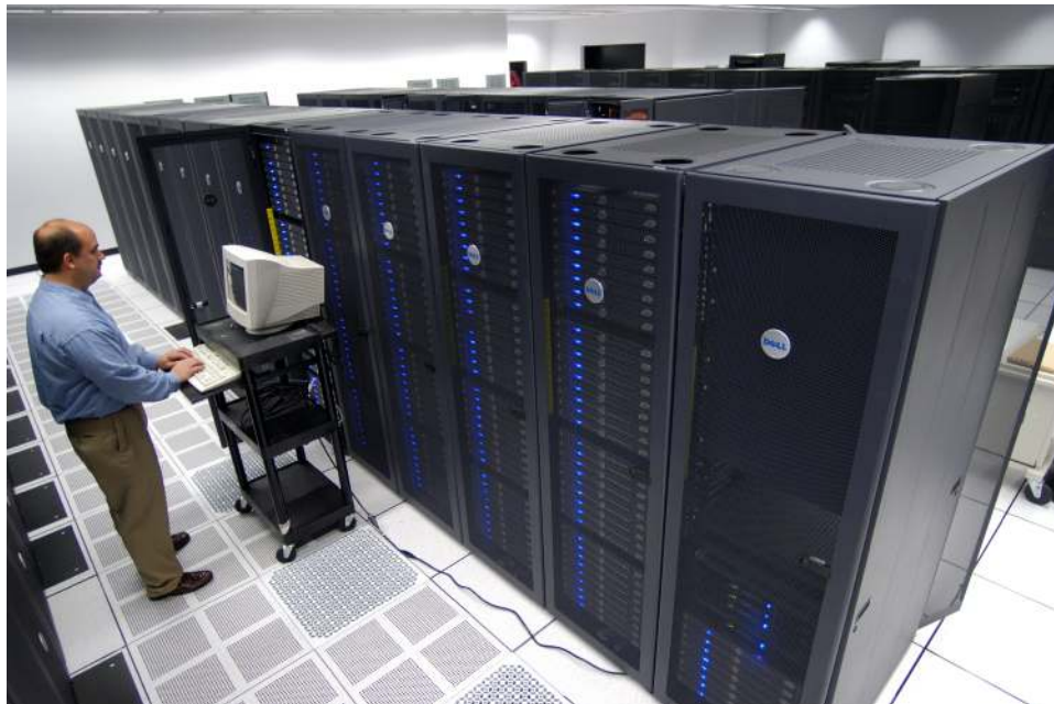
Figure 2. Cluster Built from Multiple Server Racks
