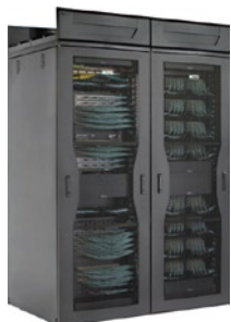
Figure 3. Panduit NetAccess Cabinet with Two Cisco MDS 9513 Switches and Associated Fiber Connectivity
