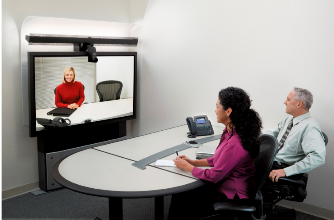
Figure 1-4 Cisco TelePresence System 1000
