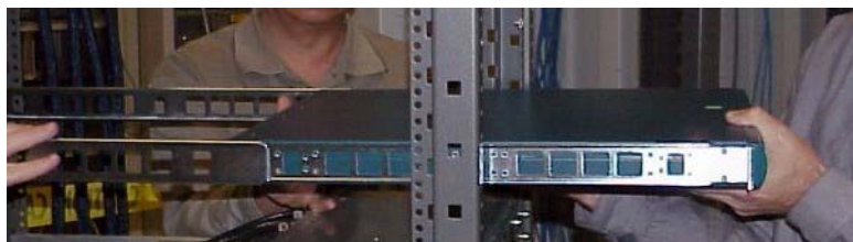
Figure 2-5: Sliding the Switch Into the Rack
