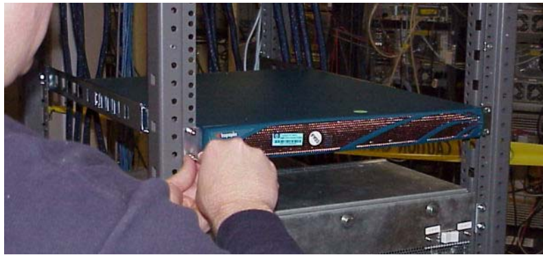
Figure 2-9: Secure the Switch Through the Front Rack Rails
