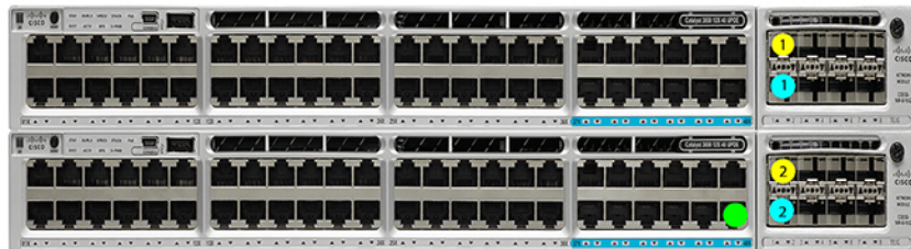
Dual 10/25GE ToR Switches (standalone or stacked)
