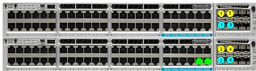
Dual 10/25GE ToR Switches (standalone or stacked)
