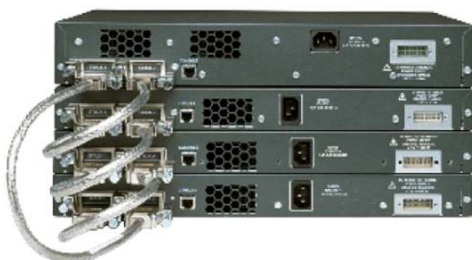
Figure 3. Cisco StackWise Technology Resilient Cabling
