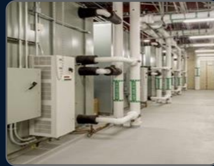
Building management systems
