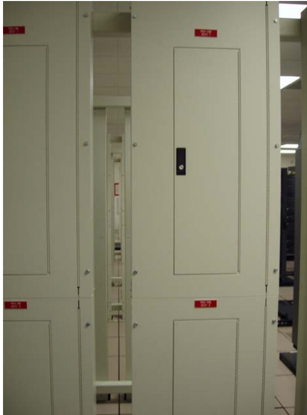
Figure 3. Power Distribution Cabinets
