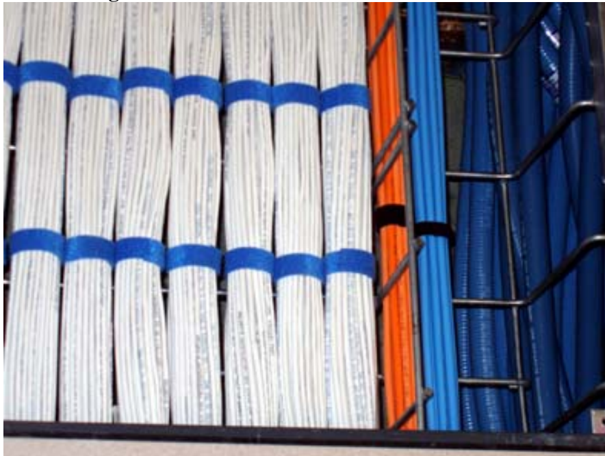
Figure 4. Cabling Under the Floor
