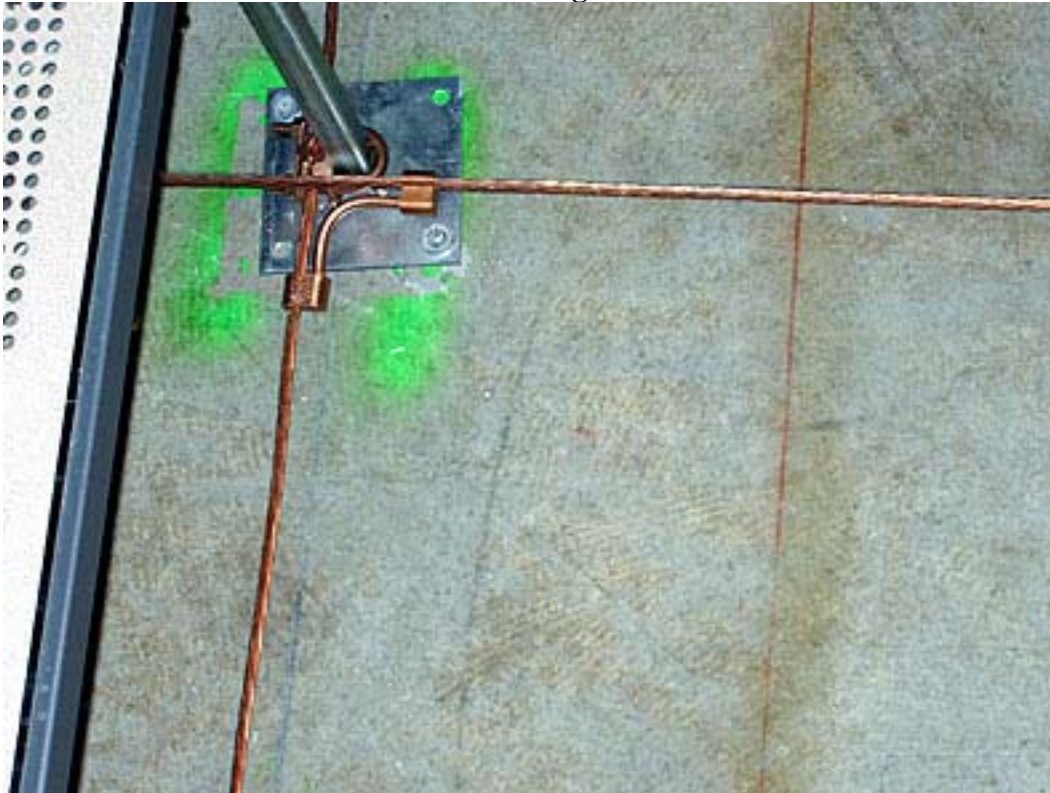
Figure 5. Close View of Power Grounding Grid
