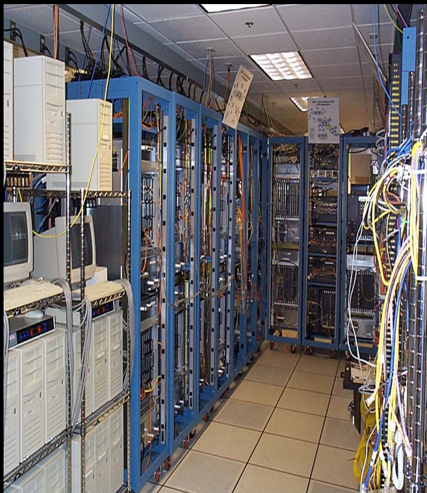
Typical portion of an end-to-end test bed
