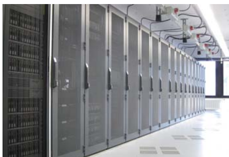
Data center, city of Pforzheim
