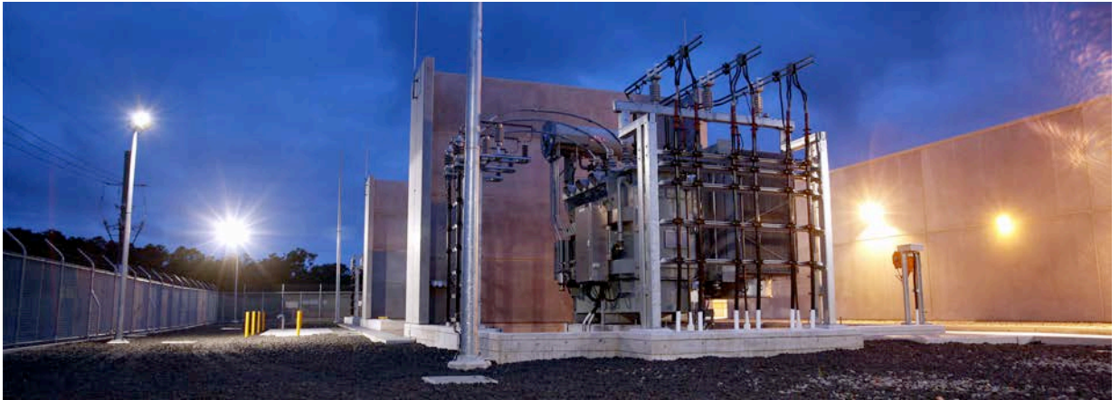
Outdoor Substation in Newcastle, New South Wales, Australia
